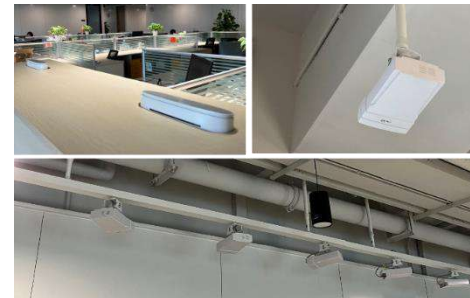
TINNO Building Indoor Wireless Gigabit Backbone Network
